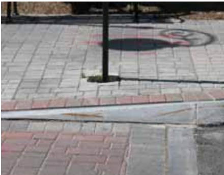
Carefully beveled granite curbs provide a smooth transition from roadside to sidewalks, and no longer challenge mobility.
